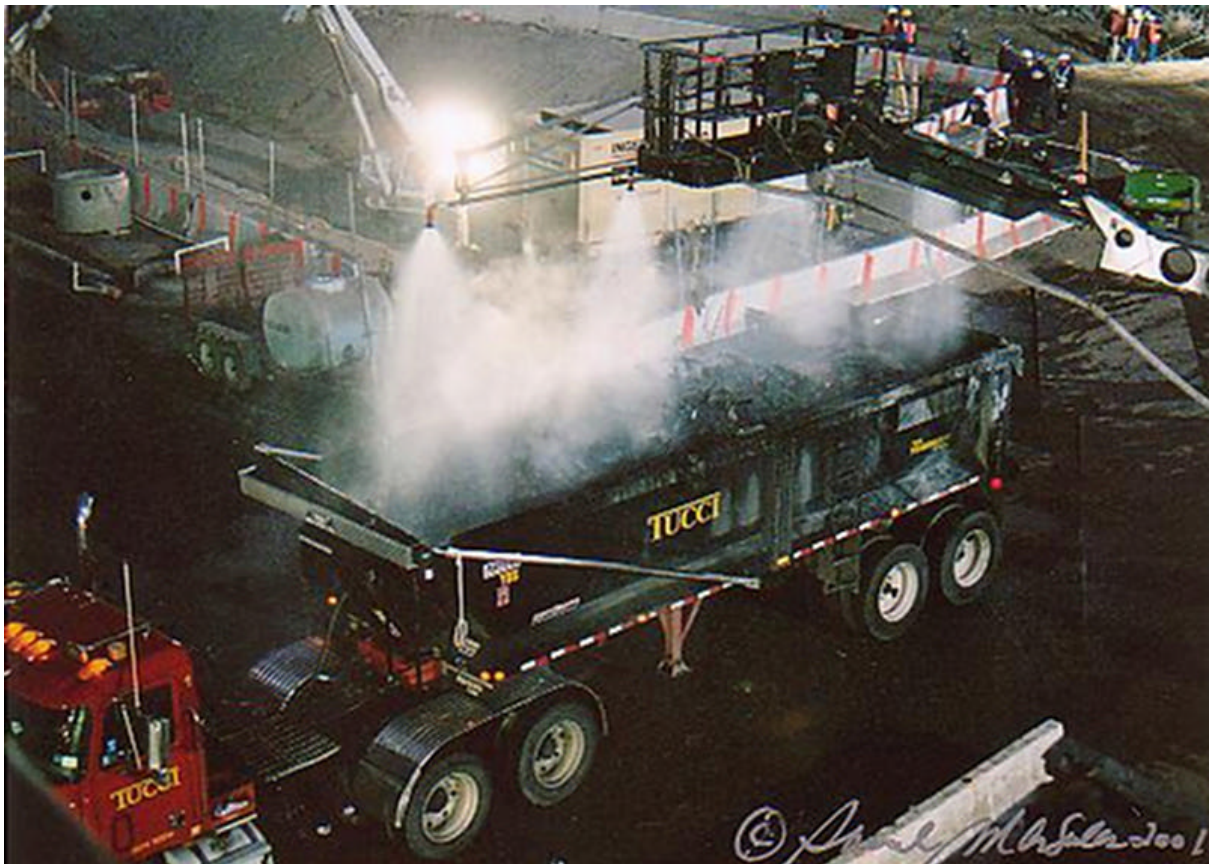
These sprayers were also used to cool the high temperature debris before it left the site. Several trucks were returned to the site for additional cooling because the law enforcement officers would not let them through the tunnels leaving Manhattan until they stopped steaming. libertypost.org/army.mil
